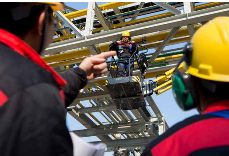
« The EPDM facility at our site in Changzhou, China, is the latest addition to our global rubber production network.
